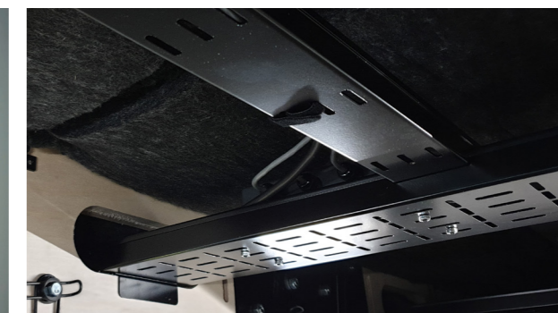
Cable-management within ceiling
